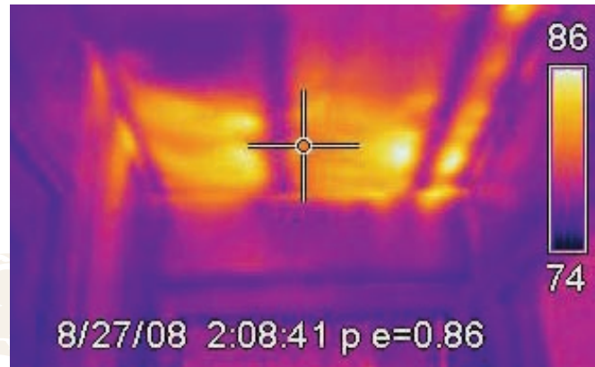
An infrared camera is used here to help detect energy leaks in this room. The orange color shows where the leaks are most prominent.
